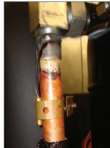
Figure 11 – Discharge Line Thermistor
